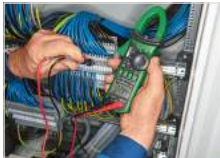
Current measurement in a control cabinet
